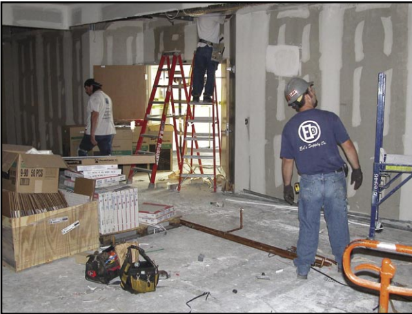
A construction crew works on the area that will be used as the main waiting room for the Myeloma Institute.
